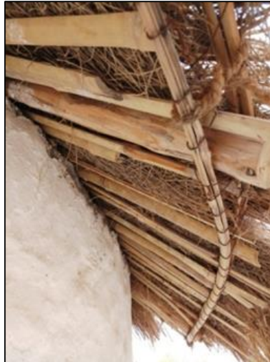
Fig. 8: Exposed Roofing material
